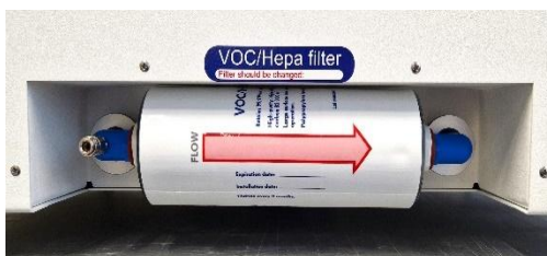
Figure 12.3 Filtre VOC/HEPA correctement installé
